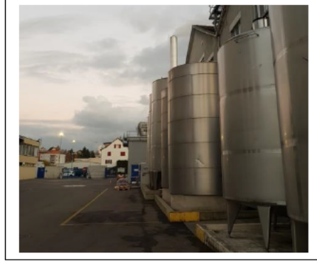
View of tank farm and discharge stack
