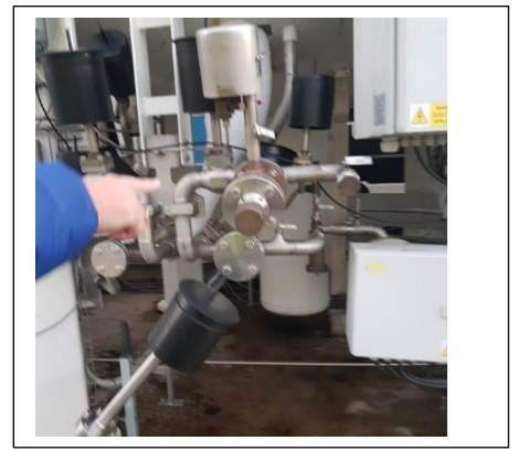
Detail of tanker connection point
