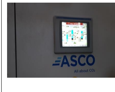
View of control panel
