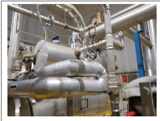
General view of reboilers for scrubbing fluid
